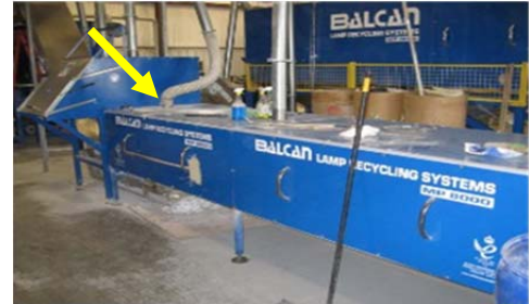
A design flaw in the bulb processing machine exposed workers to dangerously high mercury levels in the air.
