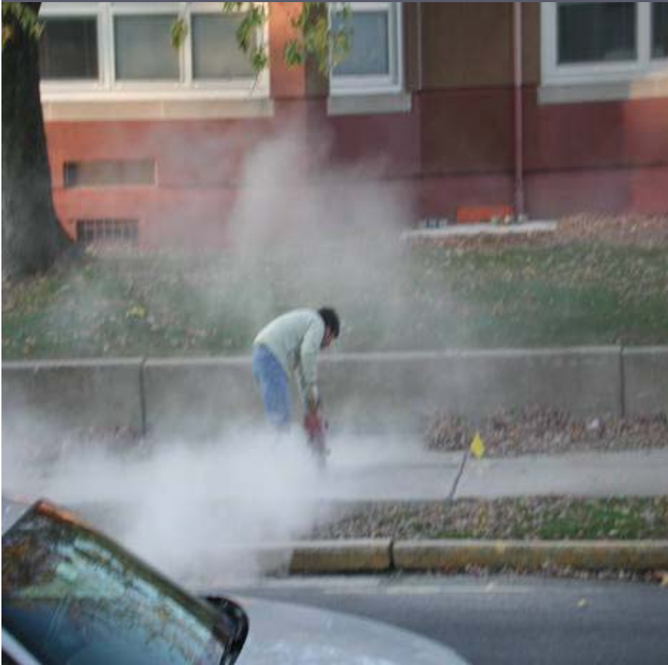
Concrete cutting using a demo or chop saw without respirator
